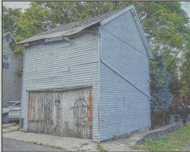
Louis Intile was granted a COA for demolishing this dilapidated garage at the back of 512 E. Fourth St. The view is from E. Morton Street.
