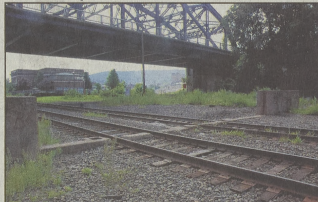
If the floodgates don't operate as intended, Union Station is the first property at risk less than a football field in length away.
