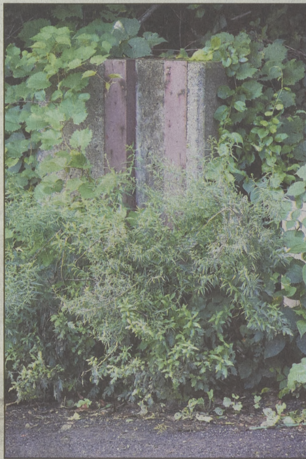
The key wall on the south side of River Drive is also overgrown.
