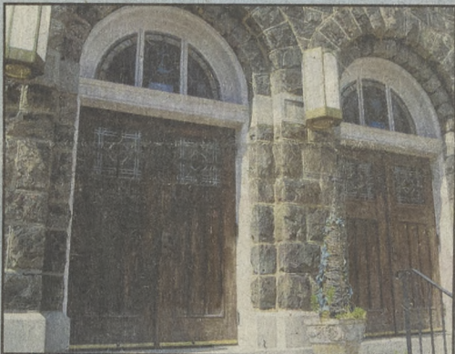
Doors to St. Joseph's Roman Catholic Church have been closed to members since July of 2008.
