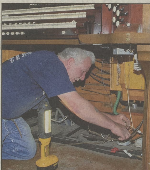
Licensed master electrician Nick Vasiliou disconnects the organ console from its power source prior to removal. Vasiliou owns NV Electric.
