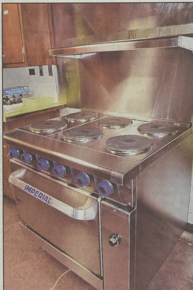
A brand new stove was installed in the club's kitchen as part of the project. A new freezer was also part of the kitchen upgrade.
