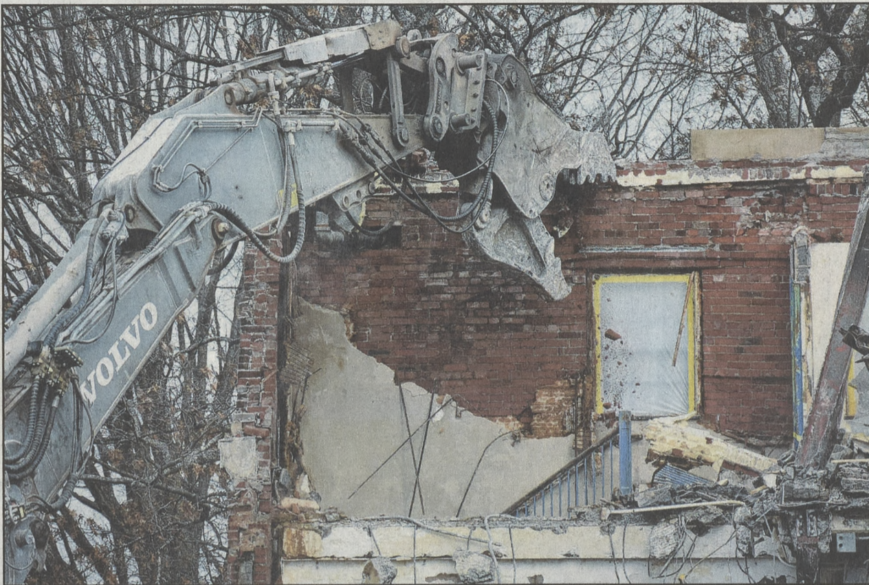
The steel jaws of a Volvo EC480EHR chew up bricks from what was once the Ritter Building where Lehigh Valley Child Care (LVCC) had its administrative offices.
