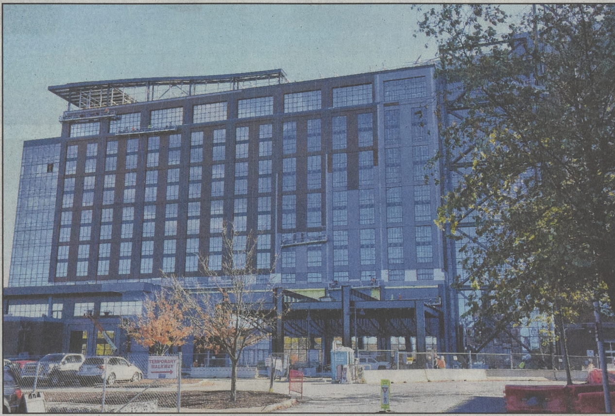
Using scaffolding, construction workers put the finishing touches on the new Wind Creek Casino Hotel tower.
