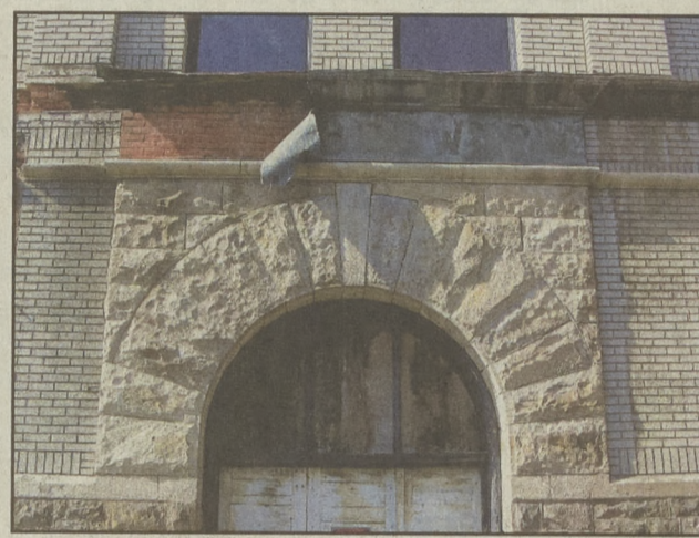
A copper brewery sign peeling away from the Miller building.
