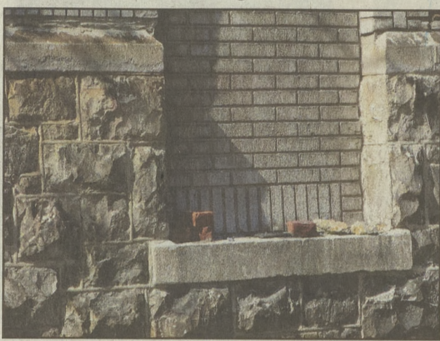
Bricks falling from the Miller building present a problem to pedestrians.
