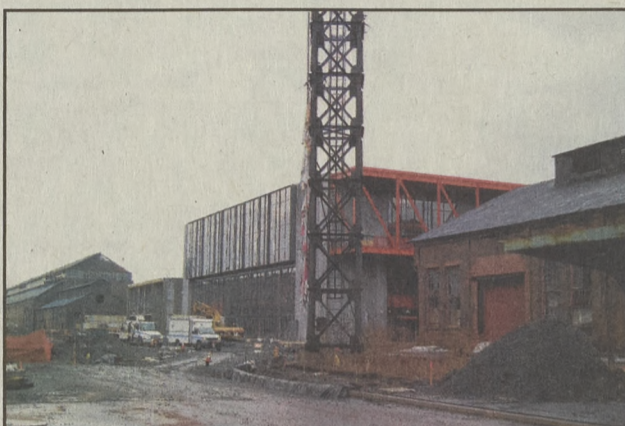
Work continues at Air Products Town Square and ArtsQuest Center at SteelStacks, First Street and Founders Way, Bethlehem.
