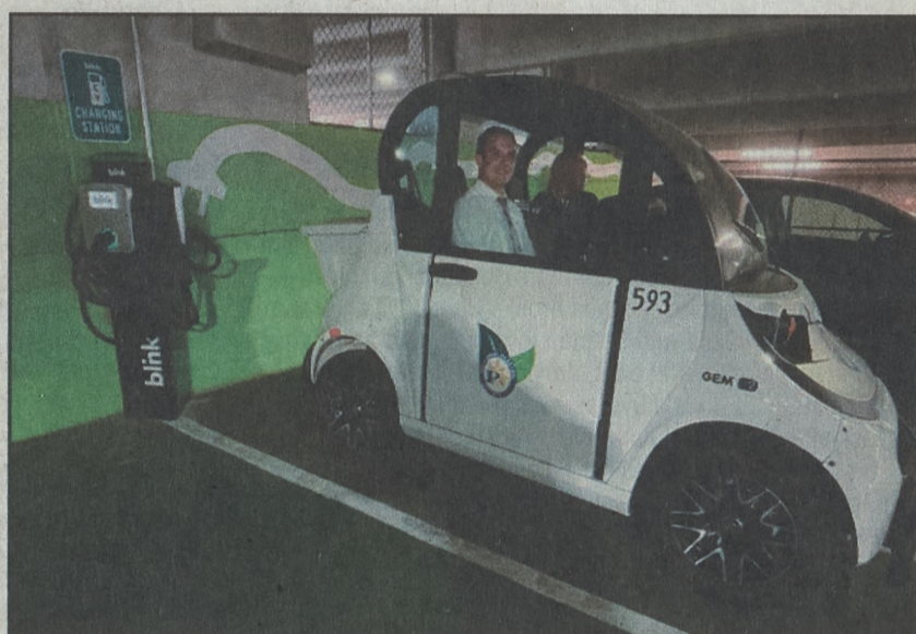
The first initiative welcomes the installation of ten Electric Vehicle Charging Stations to City of Bethlehem's Parking Authority properties.
