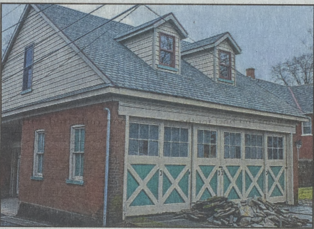
A COA was granted to replace the heavy doors facing Wall Street on this garage behind 428 High St. with a pair of overhead doors.
