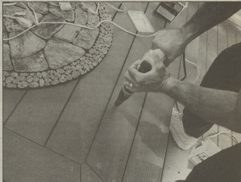
Installing a new deck may be a project best left to the professionals because of the skill level required.
