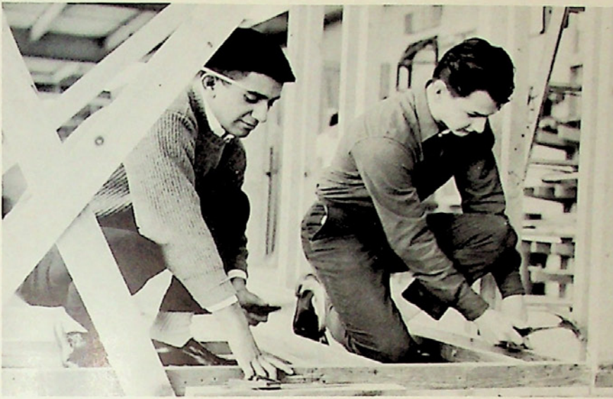
Laying a house frame engrosses Robert Cabrera and Thomas Blair during an afternoon work session.
