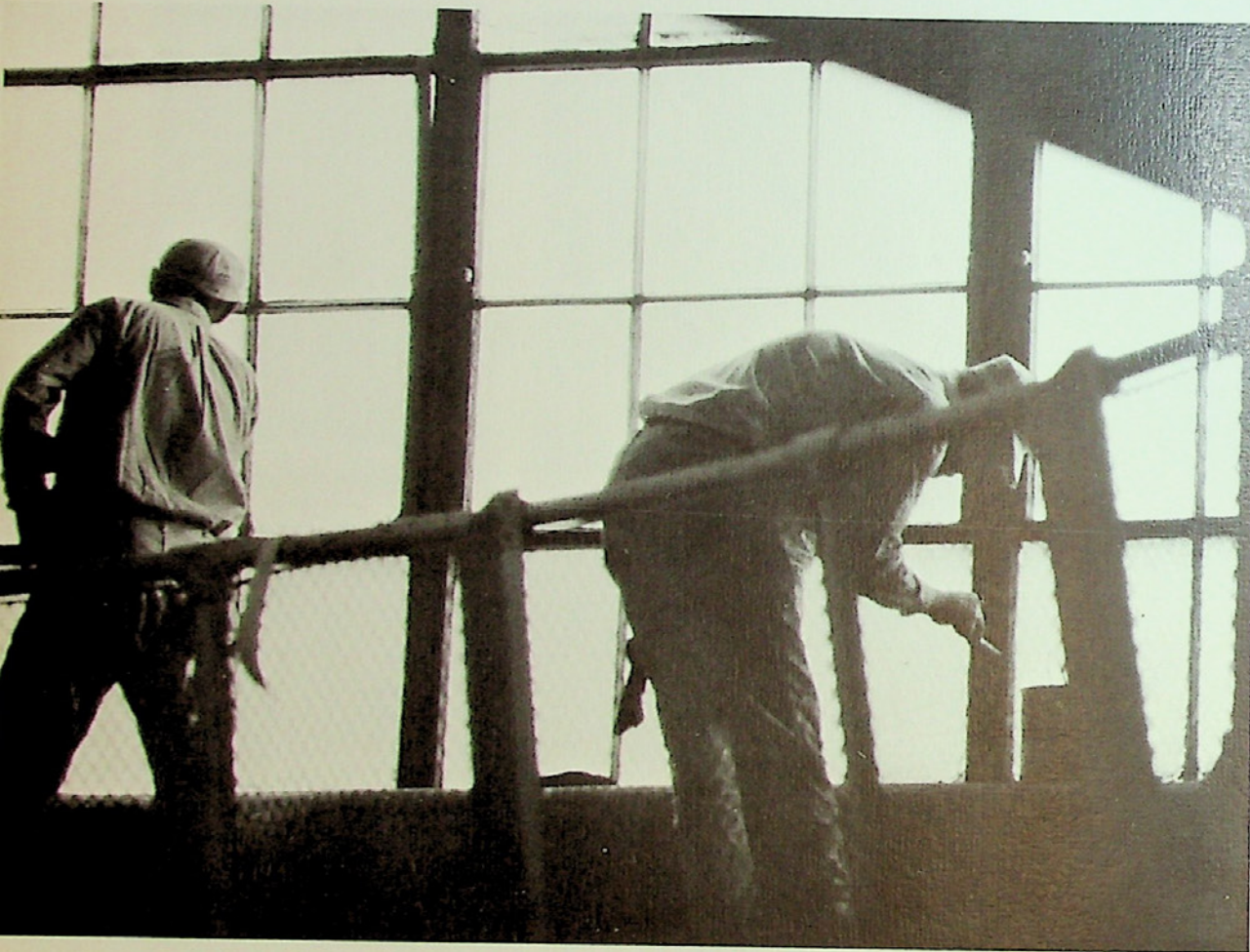
Workers on the indoor track of the girl's gymnasium give the old windows a new coat of paint.
