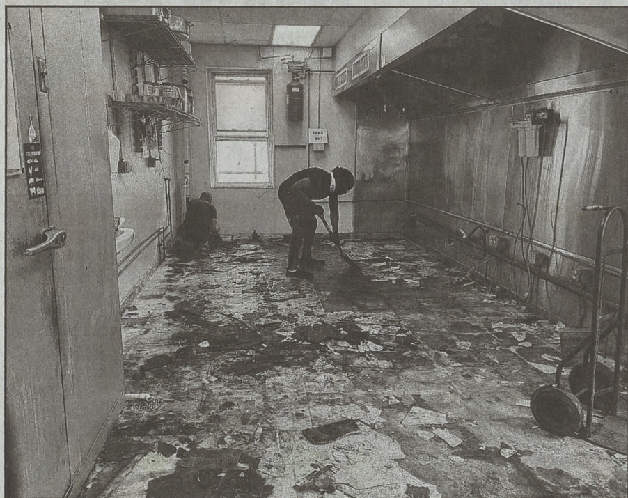
Eduardo R. and Mike W. work to remove the old flooring in the kitchen to prepare it for new flooring at the Allentown Rescue Mission.
