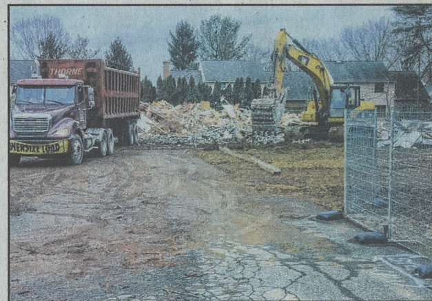
Debris from a residence that has been demolished is being removed to make way for a 61 unit apartment building.
