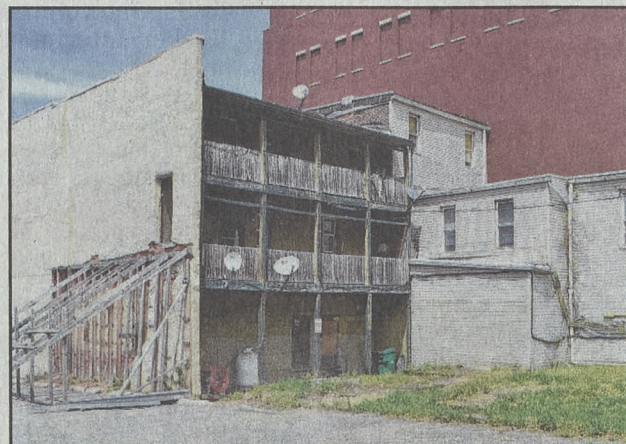
The west side and rear of 14-18 W. Third St. The deteriorated west wall is pulling away from the vacant building. A temporary wood buttress holds it in place.
