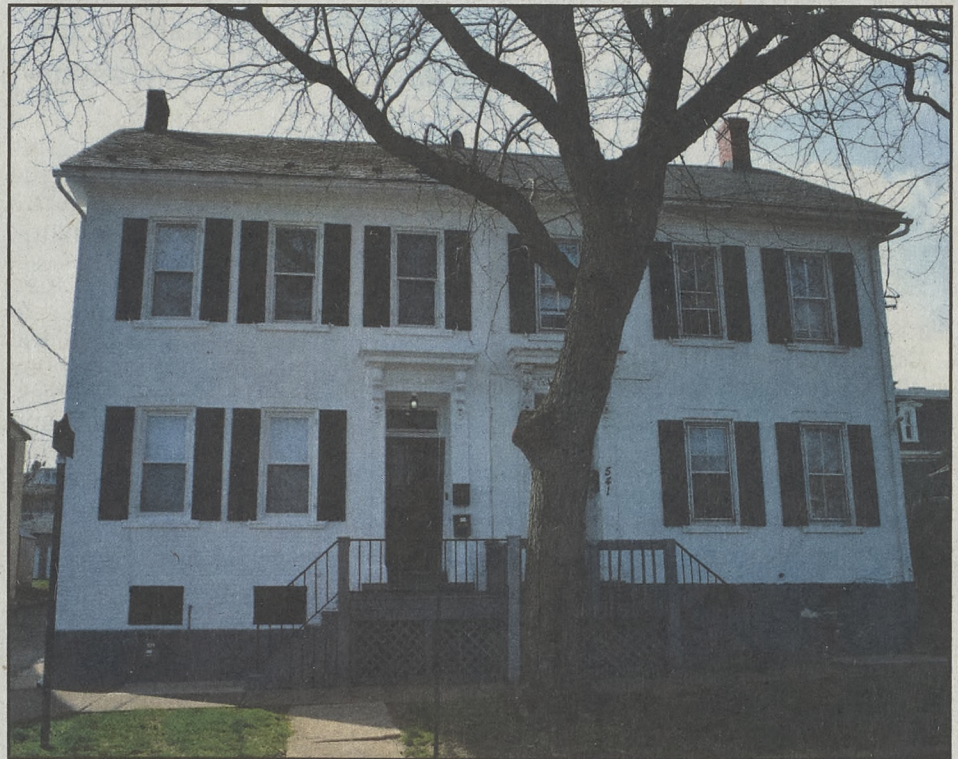
At left, 539 First Ave. was granted a COA for replacement of a deteriorated slate roof with GAF Slateline shingles to match the shingles on the other half of the twin. The roofing for its neighbor at 541 was installed in 2018.
