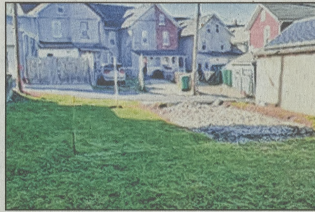
The Womer property, with a view of the old garage pad, and stakes to indicate the walls of the new garage. Mrs. Womer said the stakes were eight inches short of where the actual wall would be.
