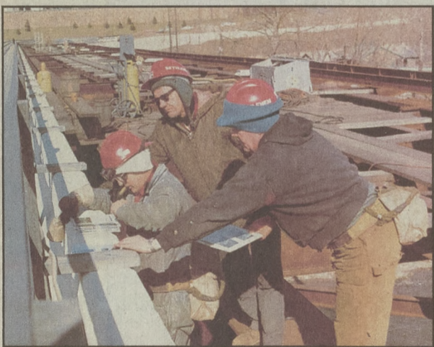
This photo of the construction of the Philip J. Fahy Bridge was taken in 1972.
