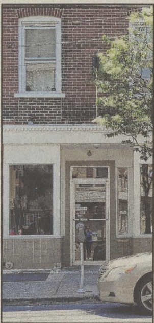
Herminio Berrios , owner of Borinquen Puerto Rican restaurant, discussed how the existing gutters leaked on his customers. The Commission granted appropriateness to the replacement of gutters on the 738 East Fourth St. property.
