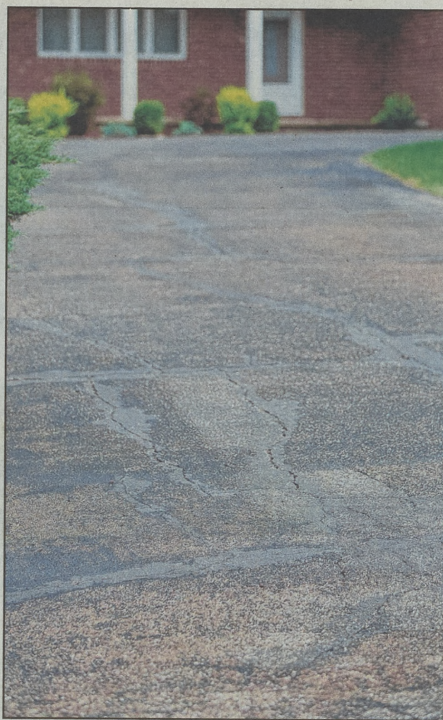
Surface cracks in a driveway may indicate a problem that requires immediate attention.
