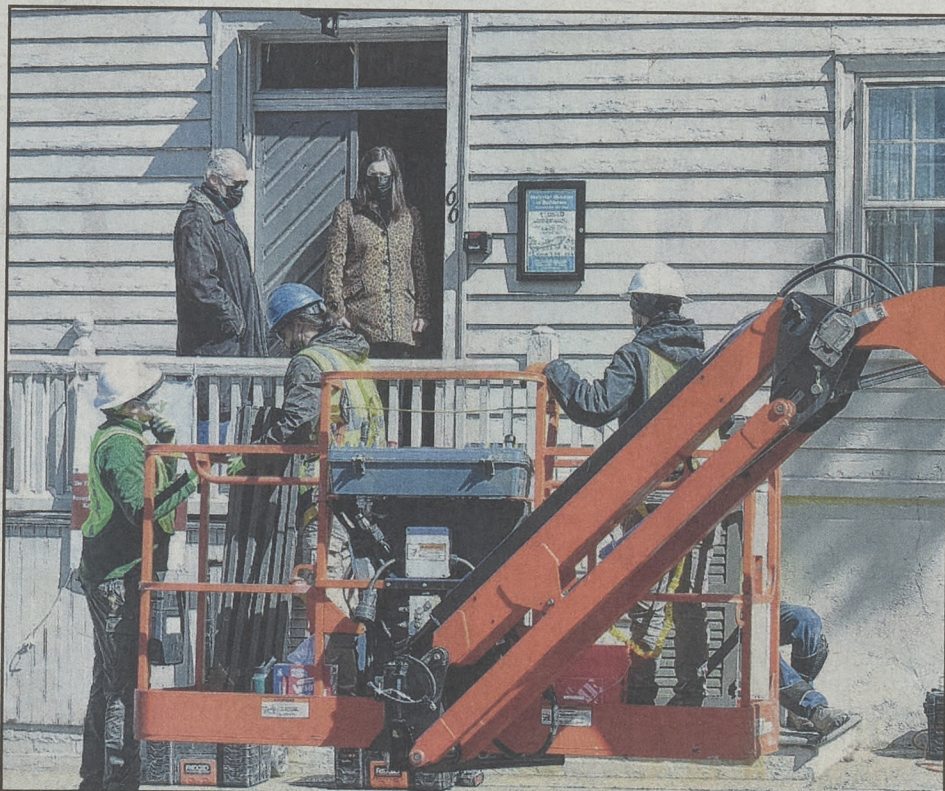
On porch, from left, are Barry Pell and LoriAnn Wukitsch, from Historic Bethlehem Museums & Sites, as they check progress while another load of shutters is loaded into the lift basket.
