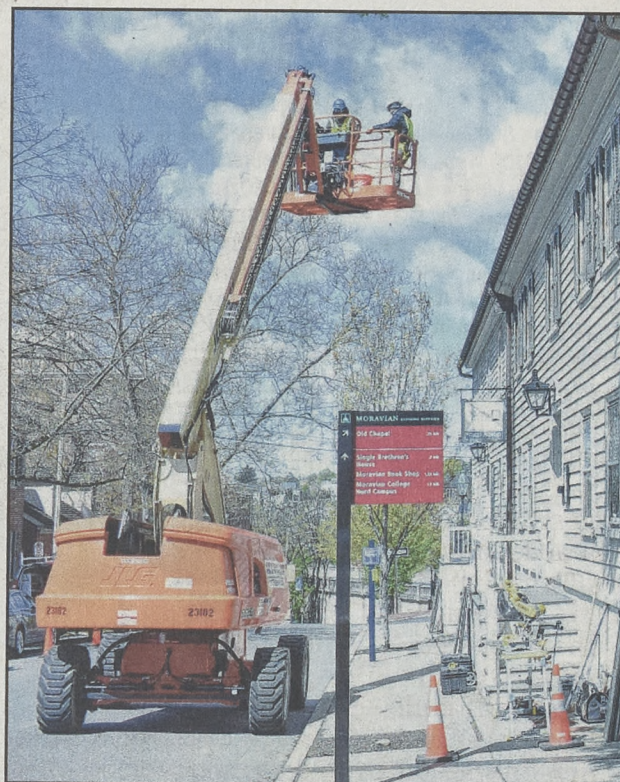
Two workers are hoisted up by a JLG boom lift with a load of refurbished shutters for installation on the second floor façade of Gemeinhaus.
