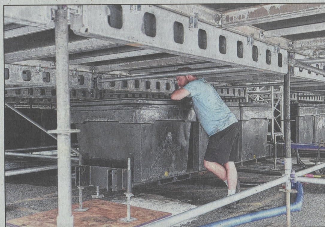
An employee of Aqua Duck Water Transport fills the ballast containers with water underneath the stage.
