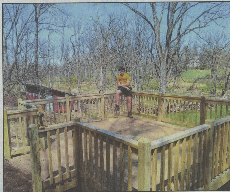
Ryan Woolley and the completed deck which overlooks a meadow and has a space cut out of the middle for a tree to grow and create a protective canopy.
