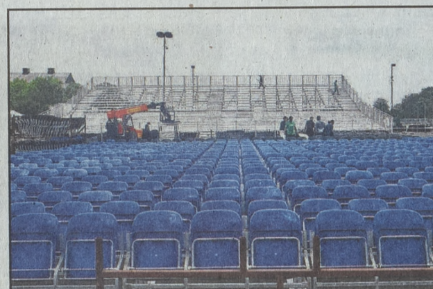
At the same time the stage is being constructed, seating and bleachers are being installed.
