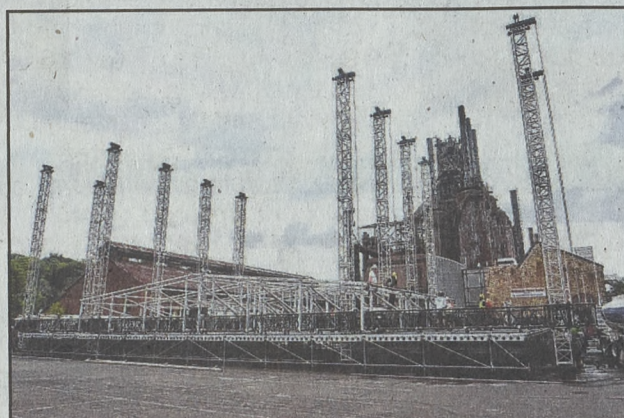
By July 28, the towers that will support the roof and other equipment rise up to the sky with the blast furnaces as a backdrop.
