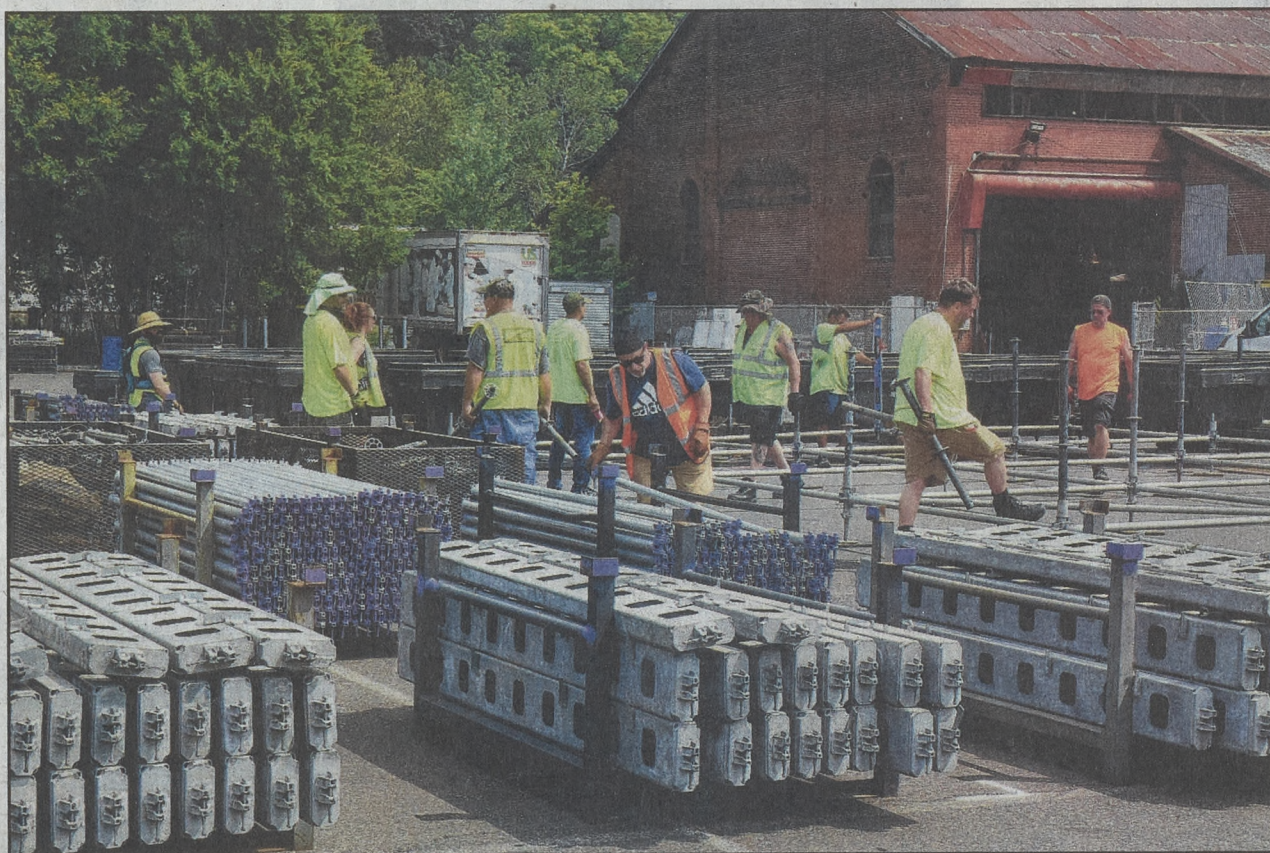
On July 25, IATSE Lehigh Valley Local 200 members begin to assemble the Tinkertoy-like components that will become the Wind Creek Steel Stage.
