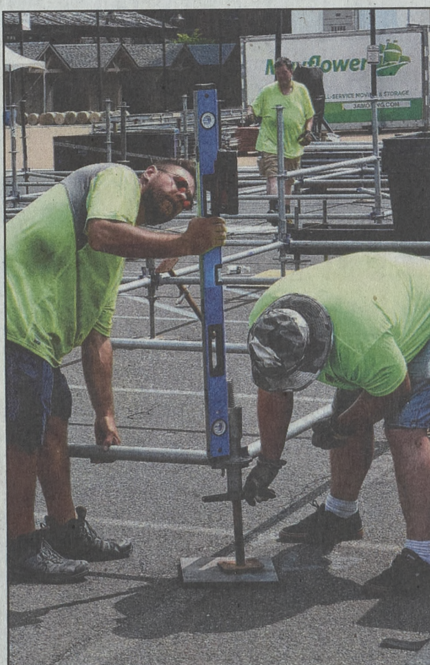
Workers begin to the process of leveling each leg of the stage.
