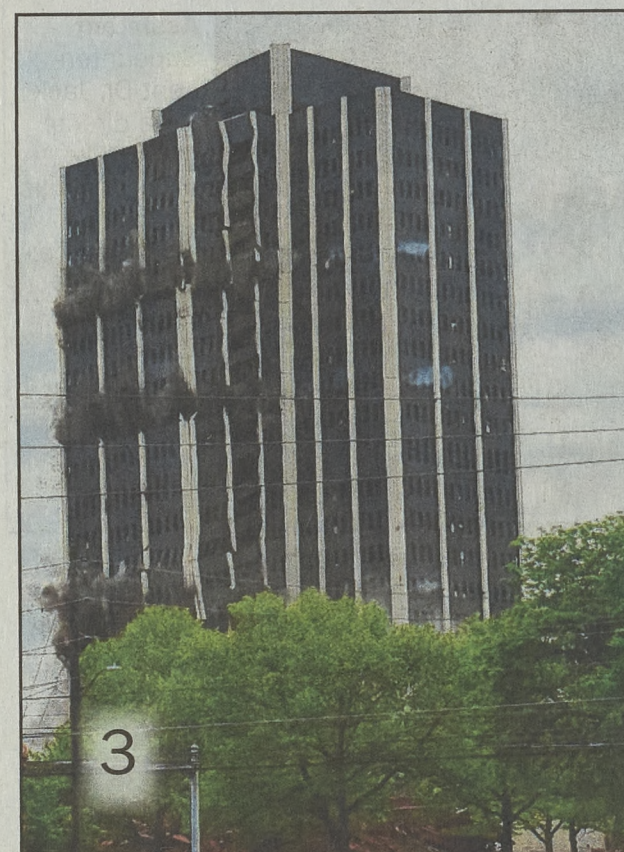
3 The eastern section of Martin Tower begins to crumple as the impact of controlled detonations affects the structure.
