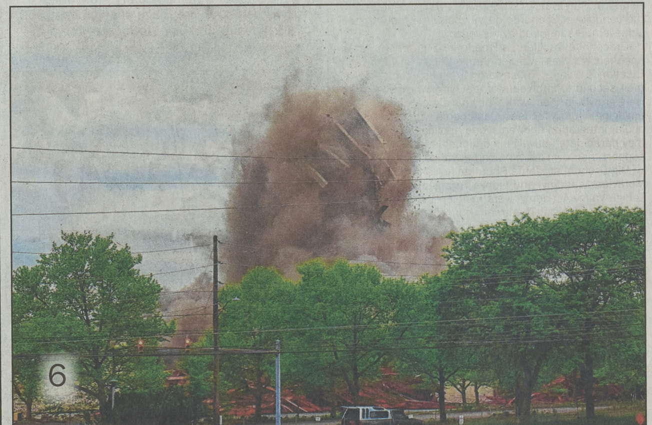
6 As debris flies, the building dissolves into a huge cloud of dust.
